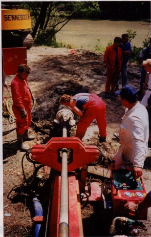
The Scorpio 903 is at its best on downtown jobs, but still able to make small river crossings like this one in Germany.
